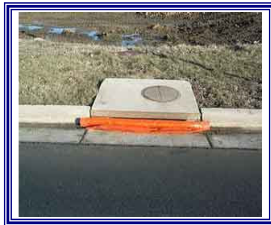
Surface Course Inlet Filter
