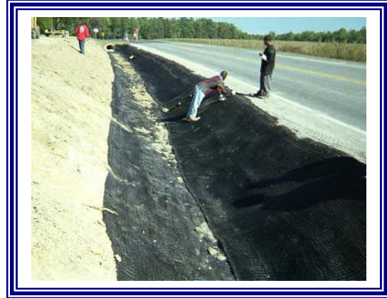
TRM Channel Application
