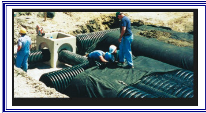
HDPE Underground Detention
