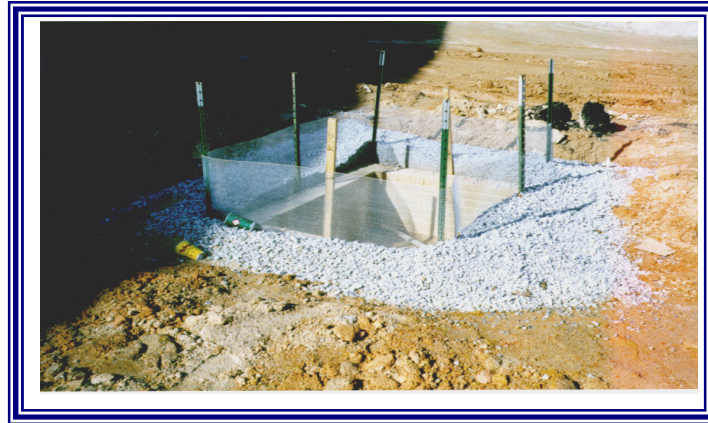
Hardware Fabric and Stone Inlet Protection
