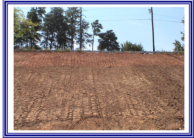
Surface Roughening (Tracking)
