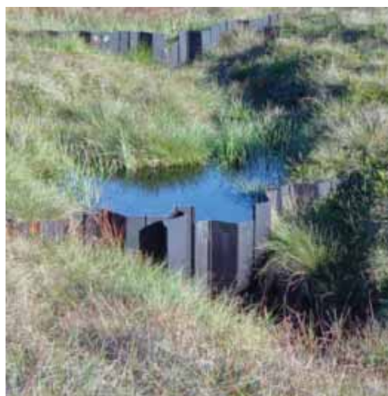
Gully blocking on peat
